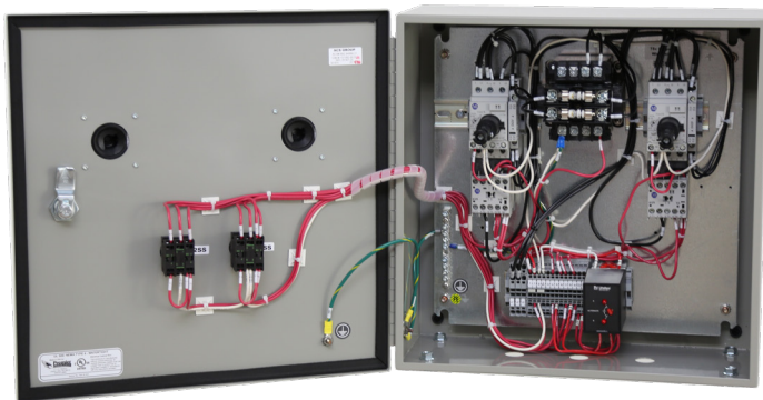
Inside view of control panel
